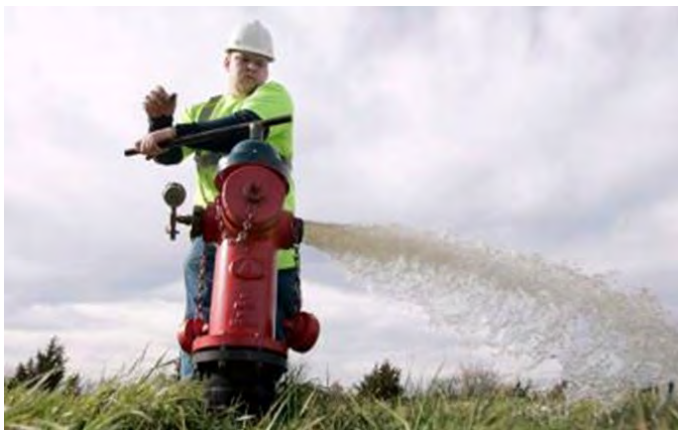
Fire Hydrant Flow Test
