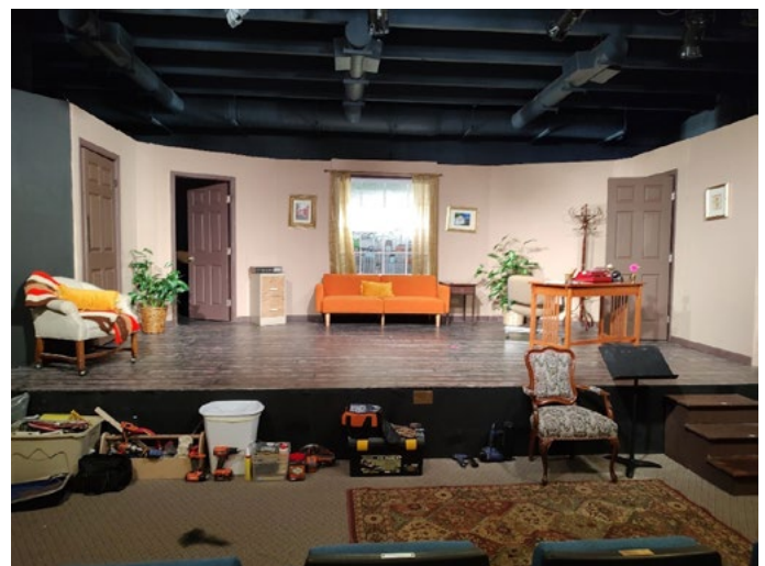
Exposed ductwork at Theatre Knoxville Downtown
