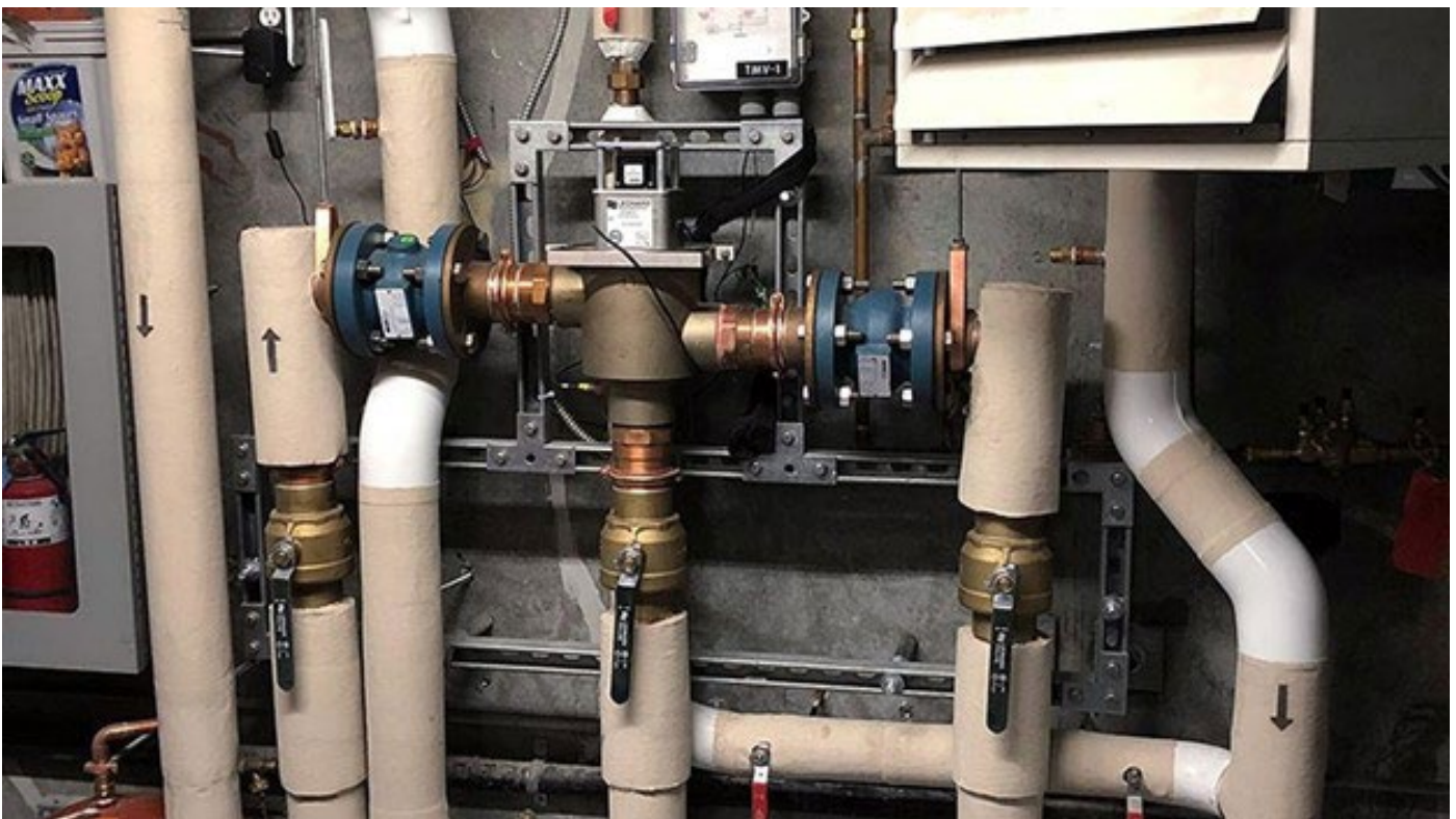
MASTER MIXING VALVE AT WATER HEATER
