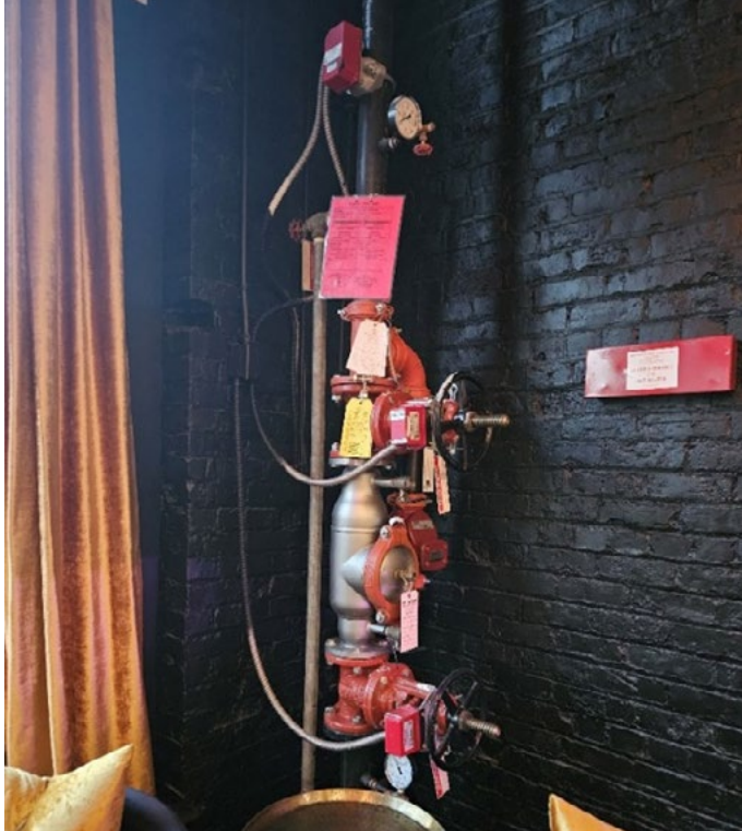
FIRE RISER WITHOUT CLOSET IN AN UN-NAMED RESTAURANT
