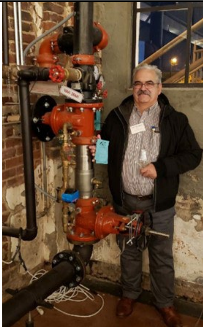
PICTURED ON LEFT, FIRE RISER WITHOUT CLOSET; ON RIGHT, GARY BERGERON
