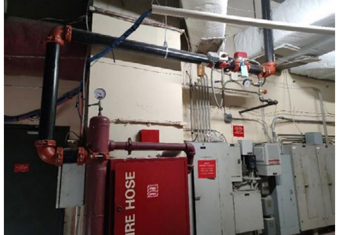
FIRE SPRINKLER AND EMPTY FIRE HOSE CABINET
